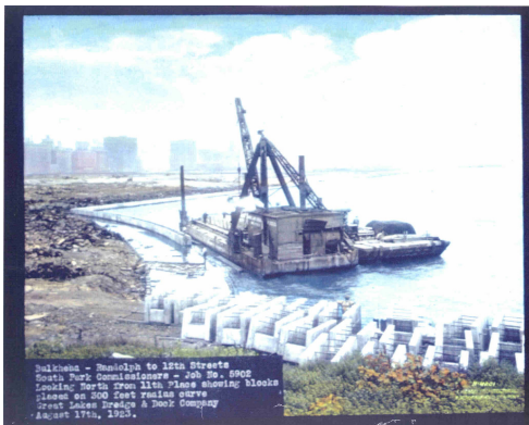
Installation of the bulkhead between Randolph Street and 12th Street. Shows limestone blocks to be placed.
