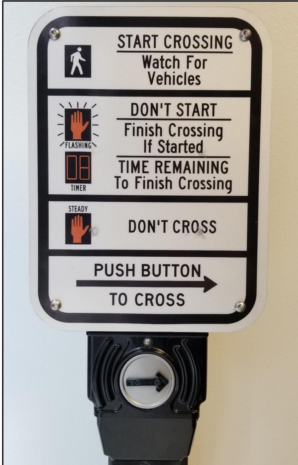
Figure 1 - APS pushbutton housing with integrated R10-3 Pedestrian Sign
