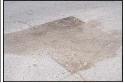
Failed utility cut
