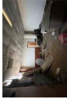
F - Buildout at north of floor and rubbish
