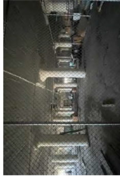
D - Chain Link Fenced Area and rubbish
