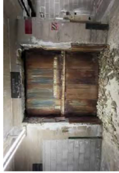
E - Elevator Lintel Deterioration
