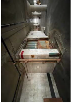
B - Damaged elevator
