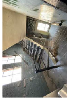
G - Stair A with cage extended from the intermediate landing of 5th to 6th Floor
