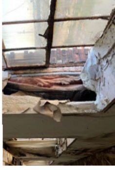
D - Deteriorated wall assembly
