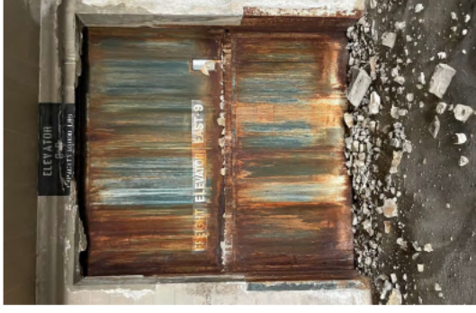
C - Deteriorated Lintel Elevator 9
