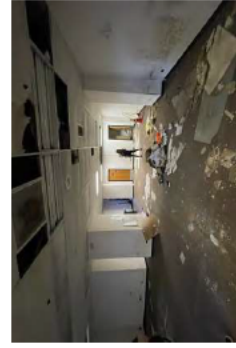
F - Office bulbout with damaged finishes at the north of floor
