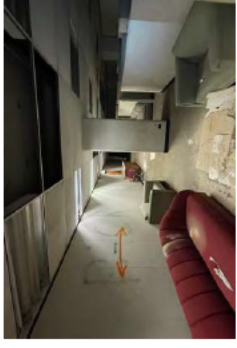
B - Interior Bulkheads and abandoned furnishings
