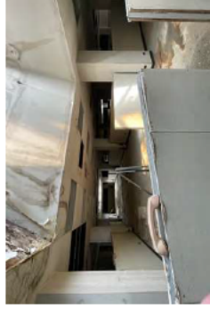
E - Partition and bulkhead, abandoned equipment
