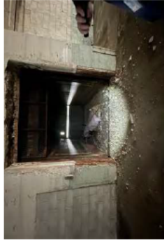
B - Deteriorated Lintel Elevator 9
