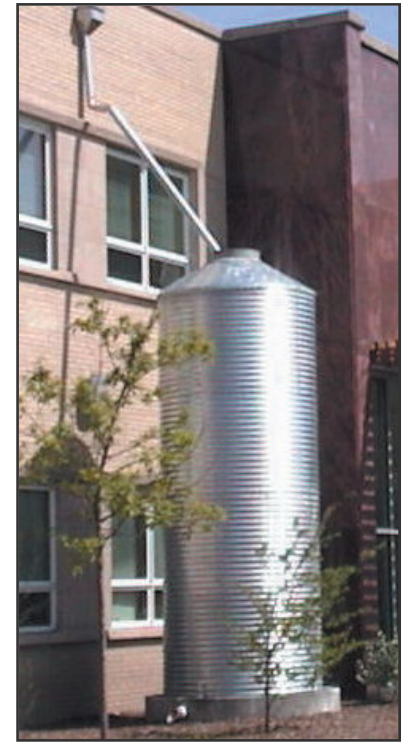
One of 4 cisterns at the Chicago Center for Green Technology (CCGT), totaling 12,000 gallons.
