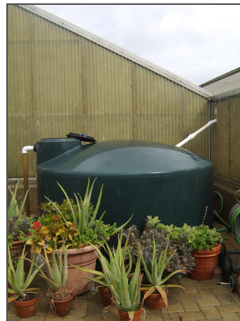
Kilbourn Park Organic Greenhouse 1,500- gallon cistern
