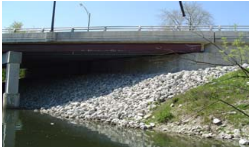
Figure 3.4 Example of riverbank with inappropriate surface treatment
