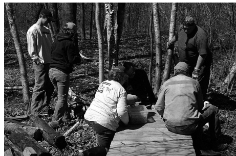
Volunteers constructing a boardwalk at Shirley Heinze Ambler Property. Photo credit: Jim Erdelac.
