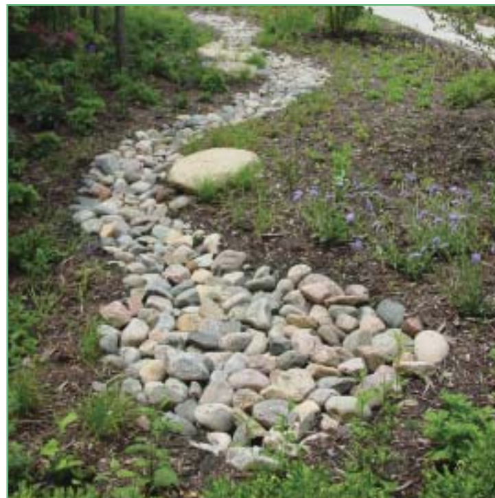
Drainage swales are one of the Best Management Practices that can effectively move water from parking and other areas.
