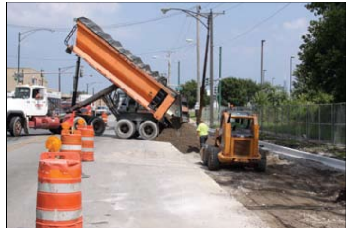
Chicago Avenue road reconstruction by the Chicago Department of Transportation. Photo courtesy of Free Spirit Media
