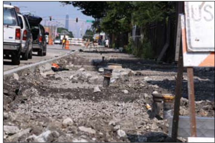
Construction on Chicago Avenue between Lavergne Avenue and Laramie Avenue. Photo courtesy of Free Spirit Media
