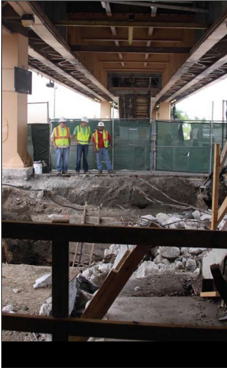
Renovation of Cermak-Chinatown CTA Red Line stop. Photo courtesy of Free Spirit Media
