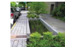
STORMWATER CONTROL MEASURES
