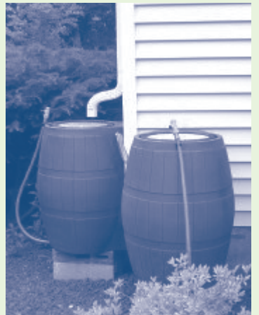
A rain barrel on cement blocks that's connected to the downspout.
